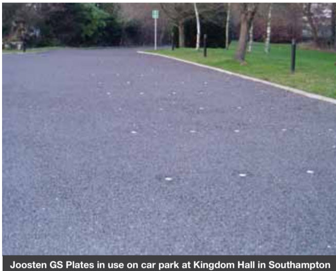
Joosten GS Plates in use on car park at Kingdom Hall in Southampton
