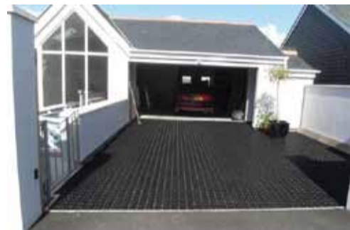
Joosten GS Plates in use on a residential development in South West England
