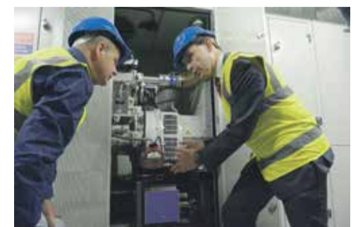
A CHP installation at a leisure centre
