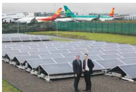
ESB CEO Pat O'Doherty at daa (Dublin Airport Authority) Solar Farm Installation
