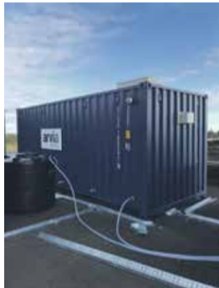
Containerised Nyex™ demonstration system on-site at Scottish Water
