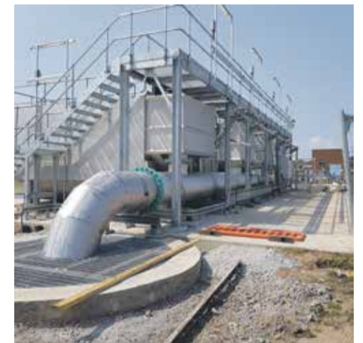
MSF 24/120 filter made up of 24 (No.) cloth filter discs with a total filtration area of 450m 2 /filter.
