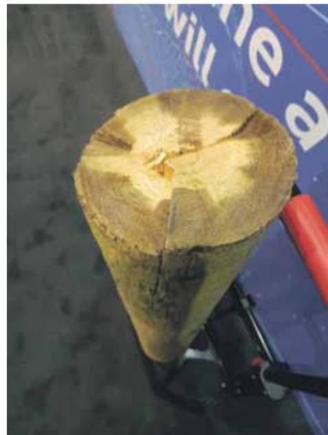
Typical problem with pressure treated poles
